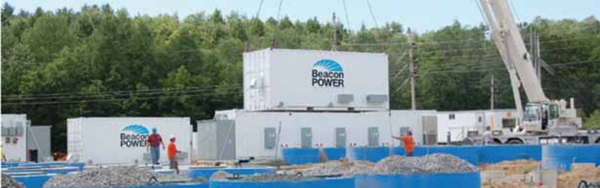
Beacon Power Corporation builds the world's first grid-scale, flywheel-based energy storage plant in Stephentown, New York.
