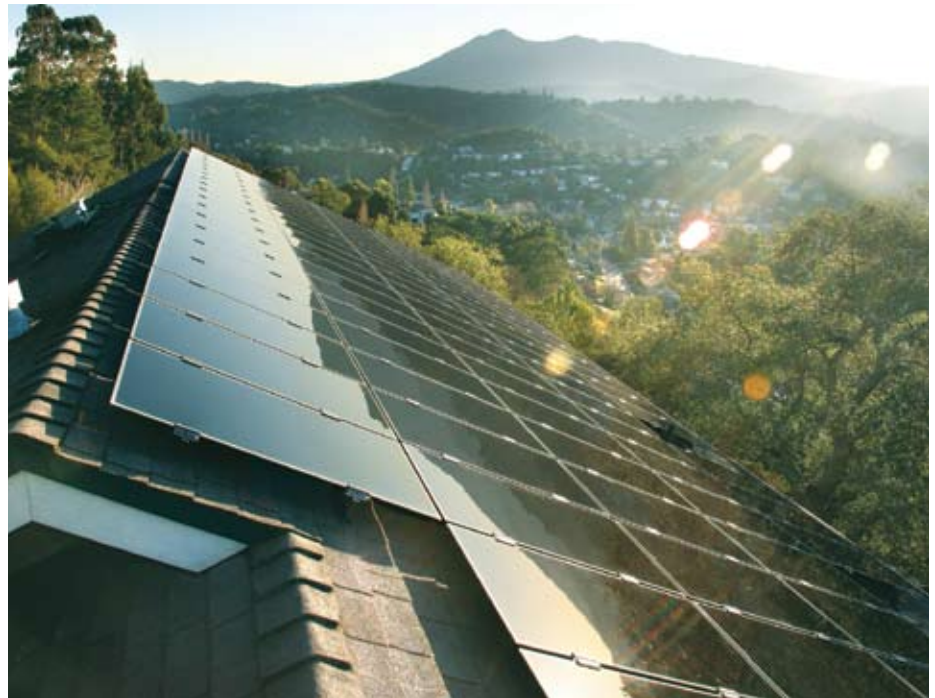
A residential PV installation in San Rafael, Calif. Photo courtesy of SolarCity
